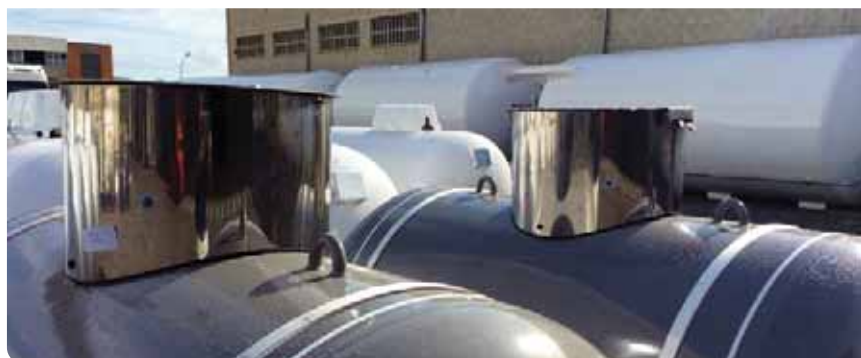
INSPECTION CHAMBERS ON UNDERGROUND TANKS
